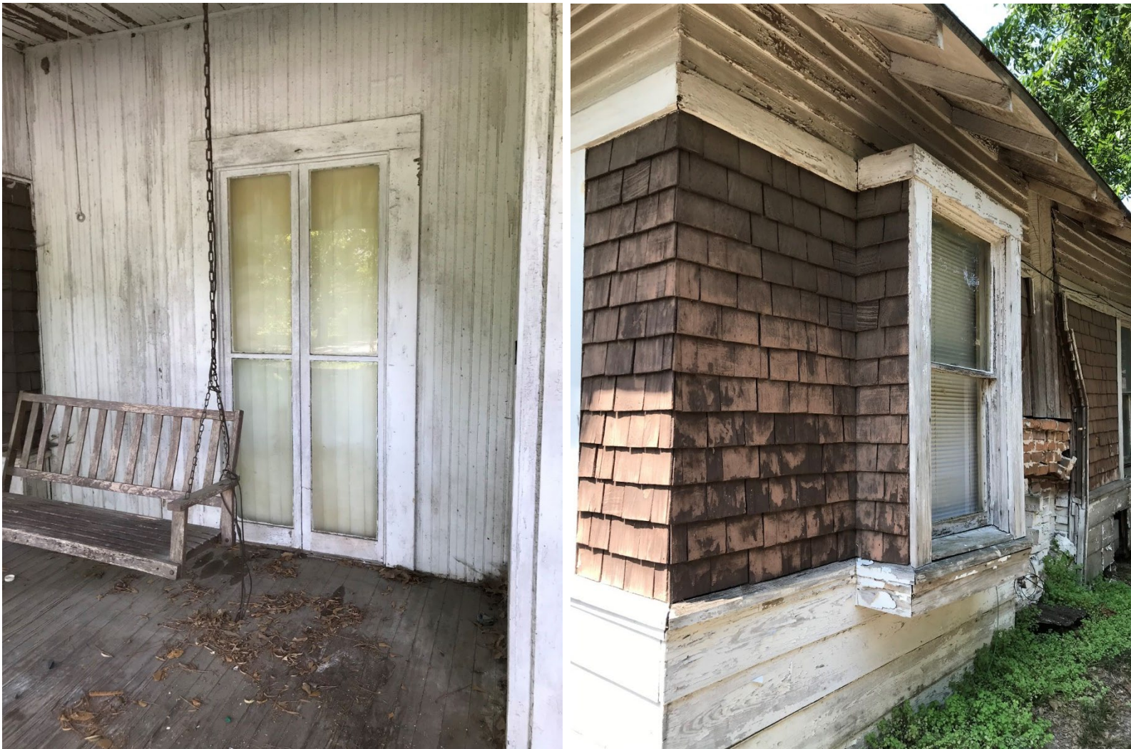
Figure 2 - Staff is requesting preservation of the window on the left is presently a condition for approval.
